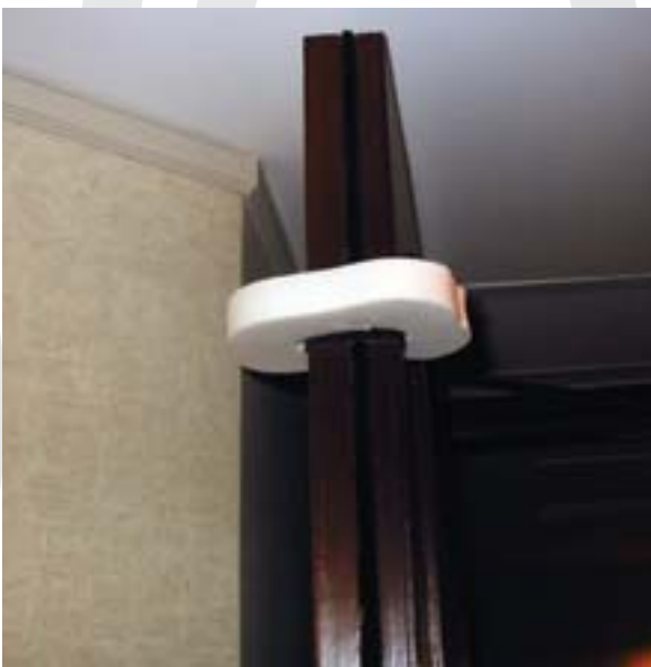
(Photo 10.2) Gasket on the entrance door in the conference room can reduce the noise emission during door closing.
