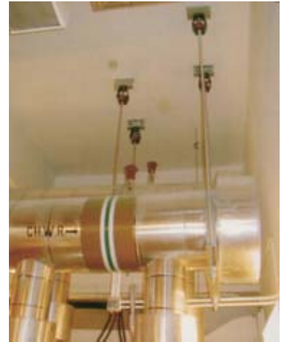
(Photo 10.3) Vibration isolators are adopted in the mechanical plant room.
